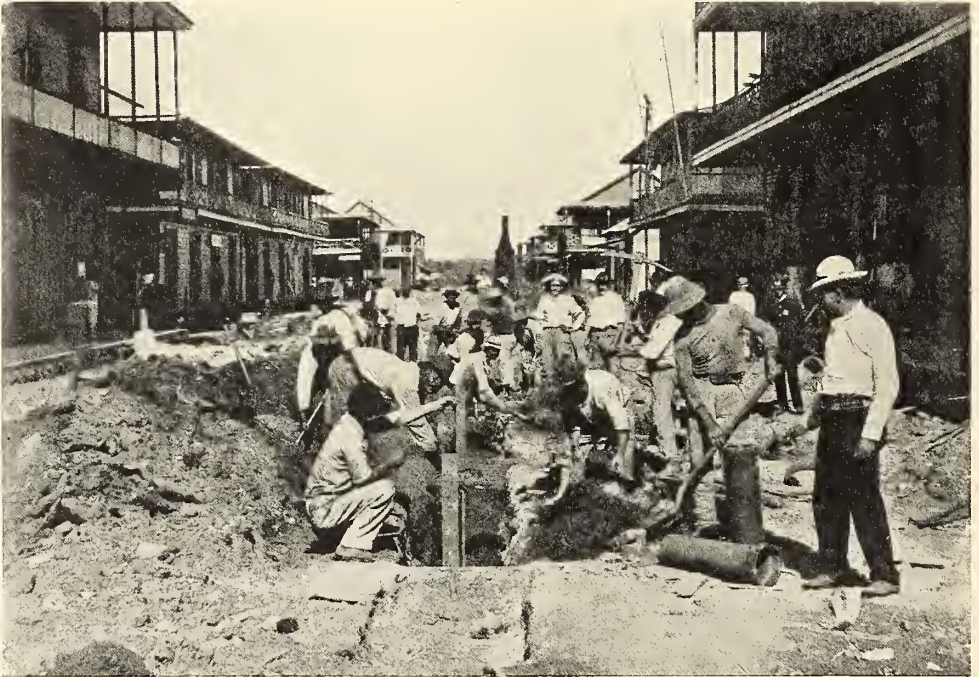
42. NEGRO GANGS OF LABOURERS AND SKILLED ARTISANS CONSTRUCTING THE DRAINAGE OF COLON (PANAMA)
